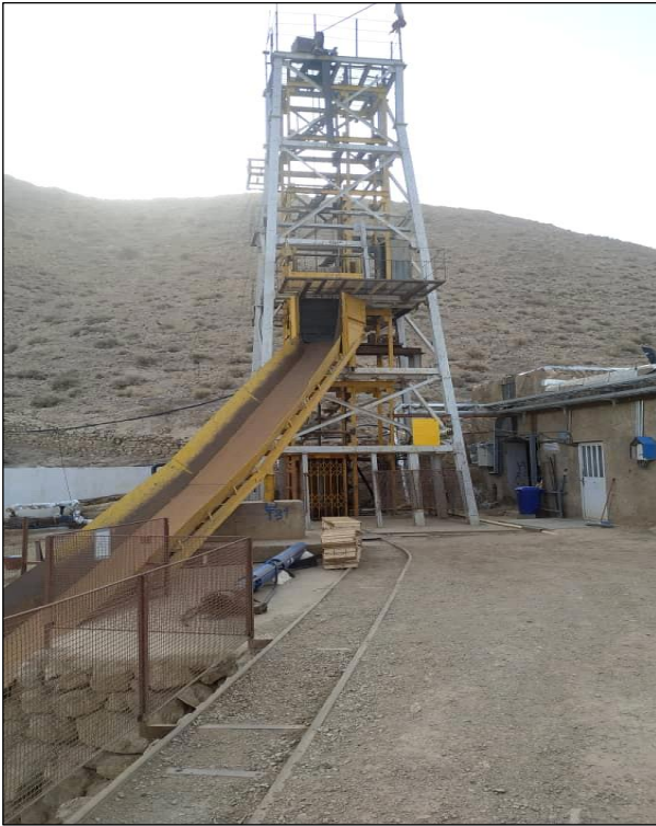
Fig. 6. Main shaft hoisting system and equipment in the Tajkuh mine
